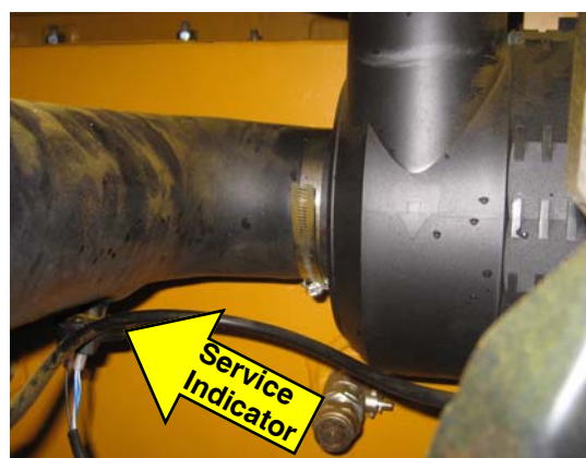
7: Check air filter indicators at ignition box (water/fuel light)
